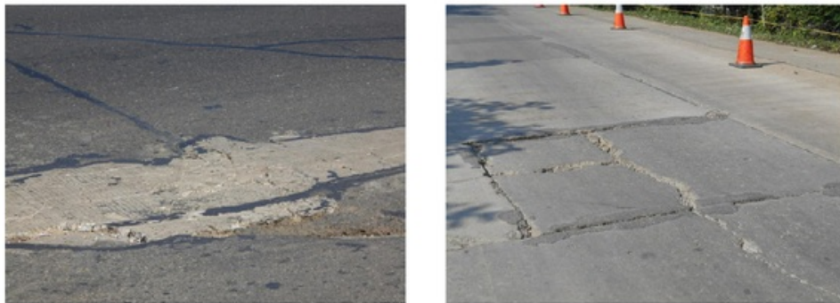
Fig. 1. Damage to the rigid pavement.
